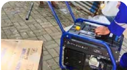
Uji coba genset Generator Trial
